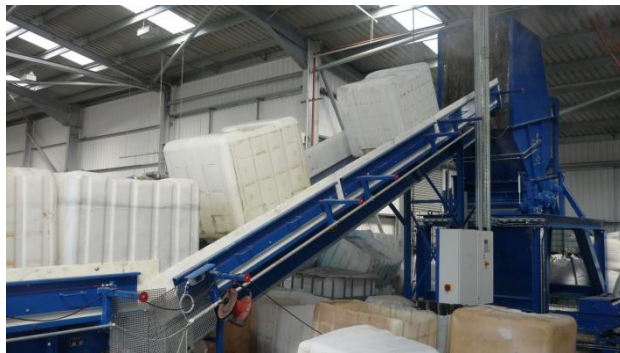
Plant for shredding IBCs at TDG in England
