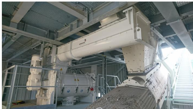
Shredding plant for substitute fuels sample analysis
