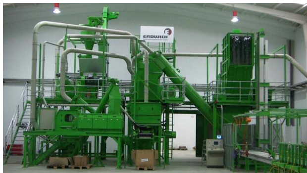
Efficient reprocessing of old cooling units in Spain
