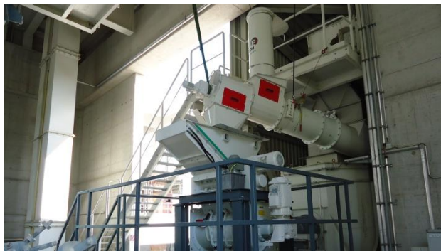
Shredding plant for substitute fuels sample analysis
